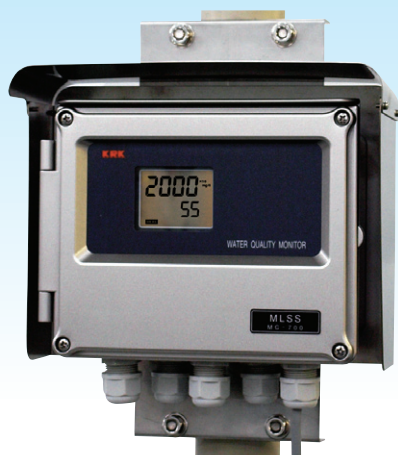
Measurement of activated sludge density in the aeration tank
